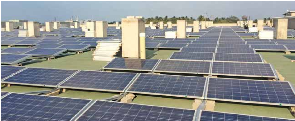
→ 1,596 solar panels installed at Viva Wajiira on the 5,000 km 2 of rooftop terrace to capture sunlight.
