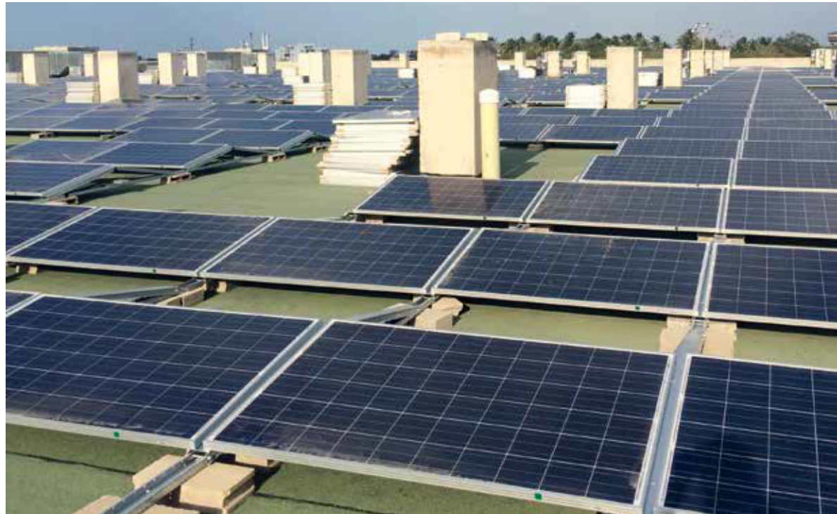
|| Éxito Panorama's photovoltaic power plant in Barranquilla has 2,070 solar panels.
